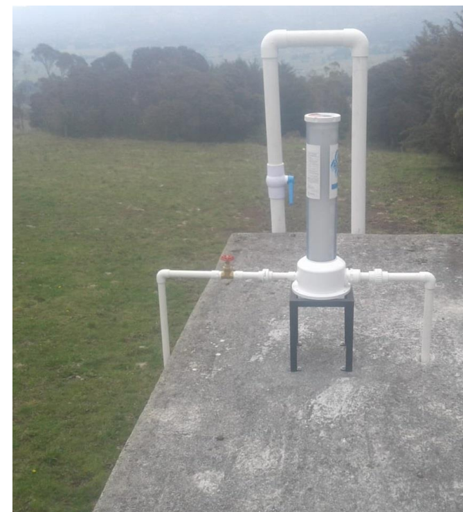
CLORADOR ACCU-TAB – TANQUE No. 3, ELEVADO
